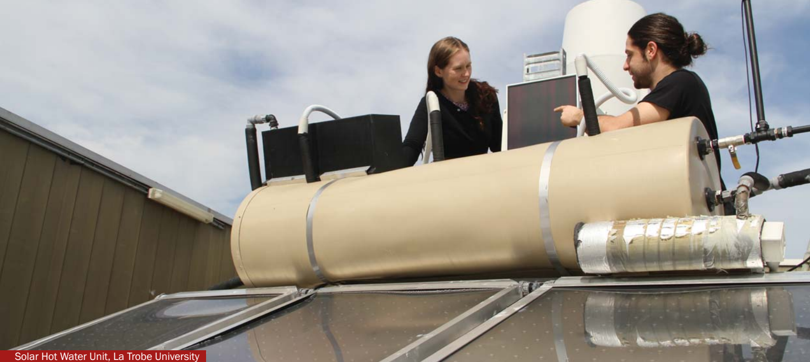
Solar Hot Water Unit, La Trobe University
